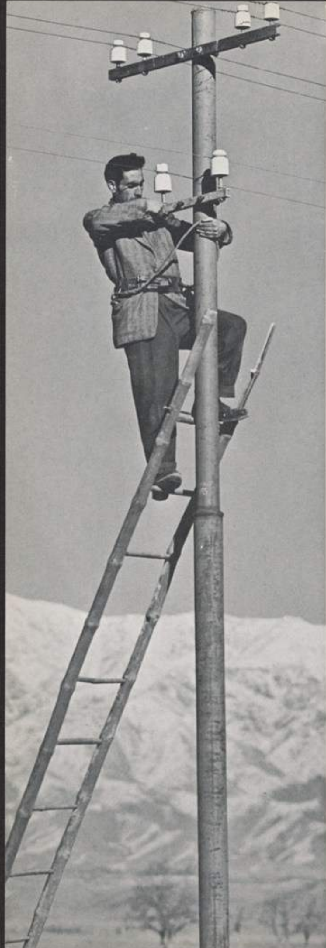
Telephone lineman at work on Kabul-Kandahar circuits. Number of telephone workers has increased nearly 30 per cent in last five years.
