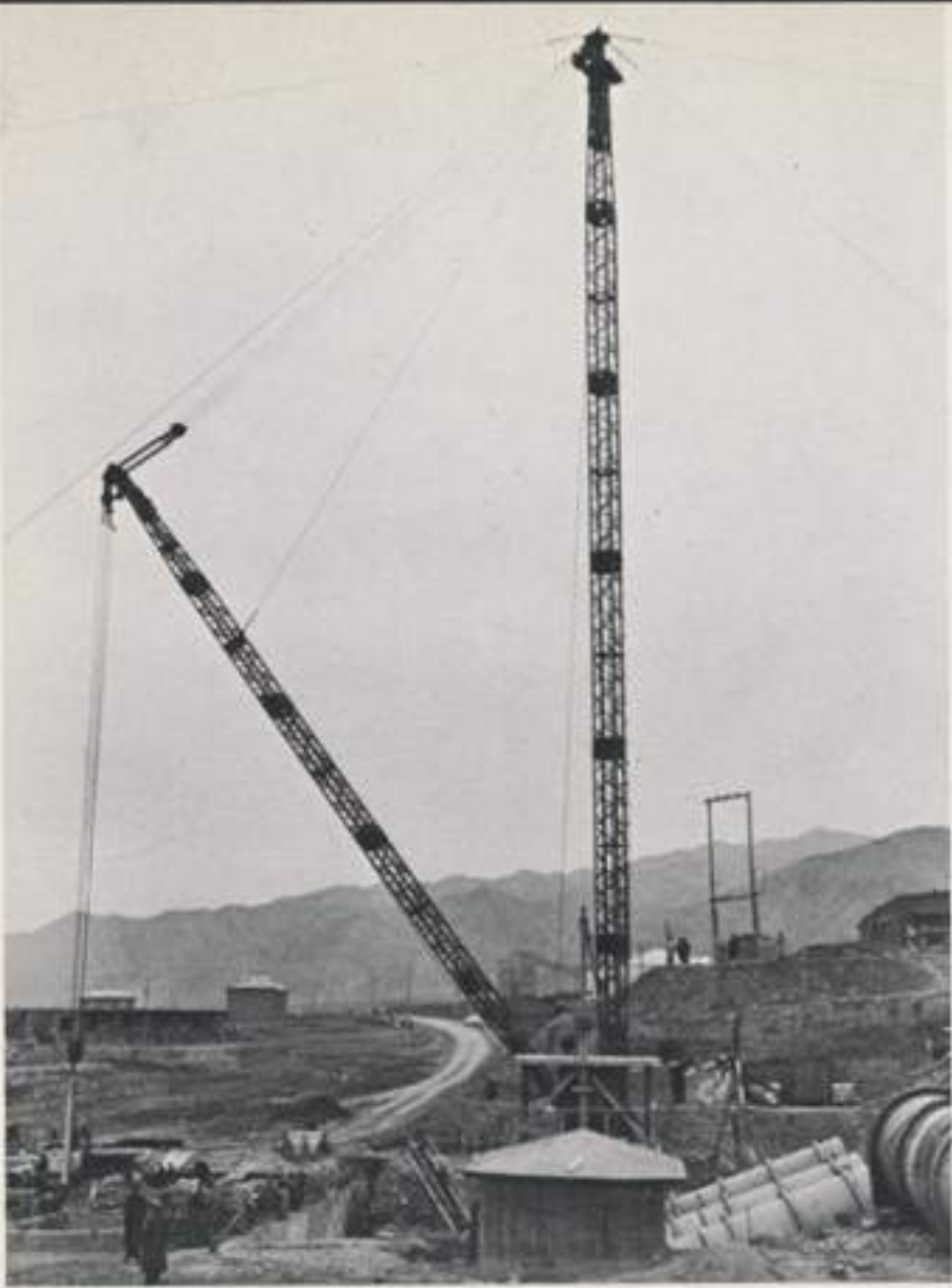
The Ghorī hydro-electric plant.
