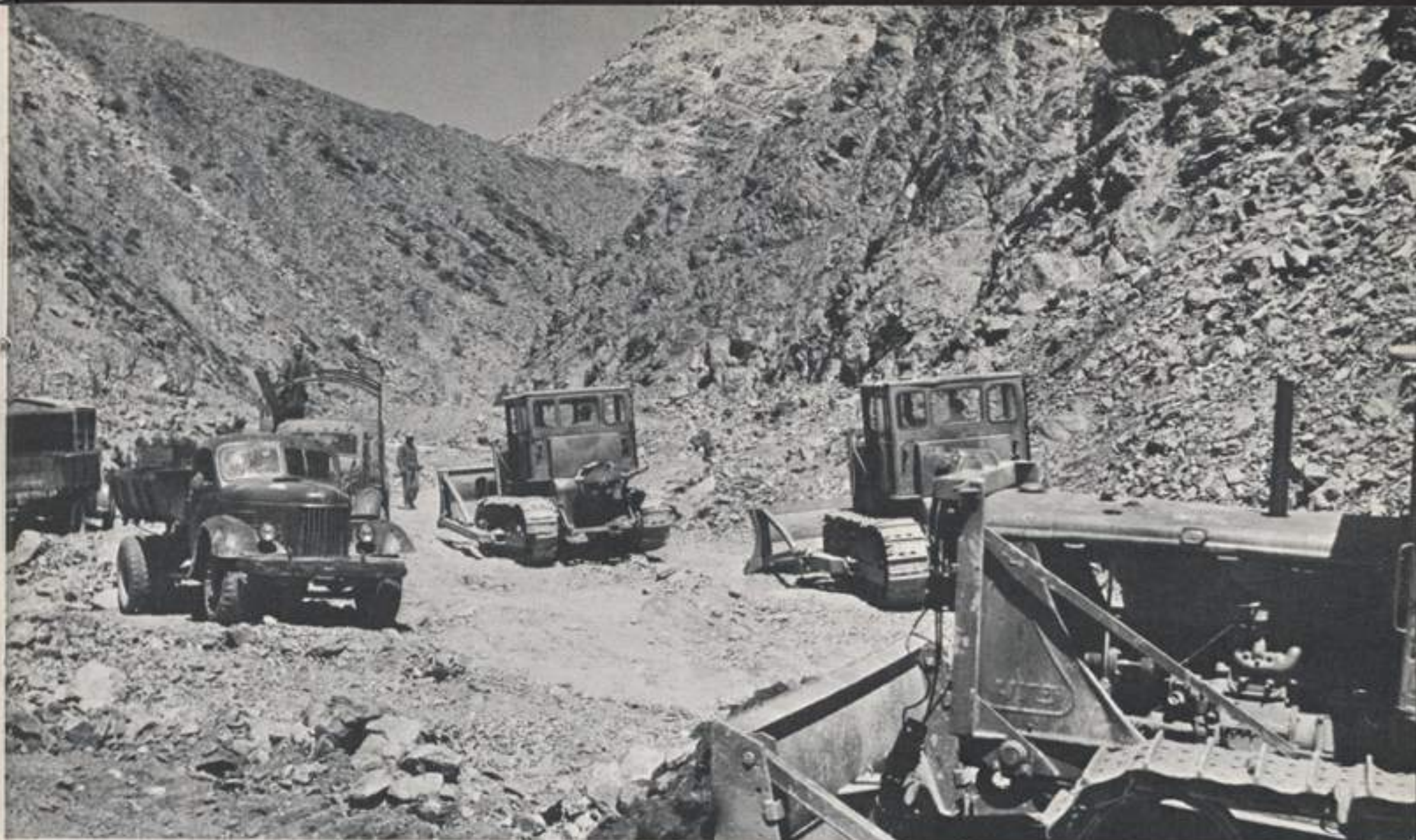
The 2 1/2 kilometer tunnel through the Hindu Kush mountains at Salang will shorten the route to the north by 200 kilometers.
